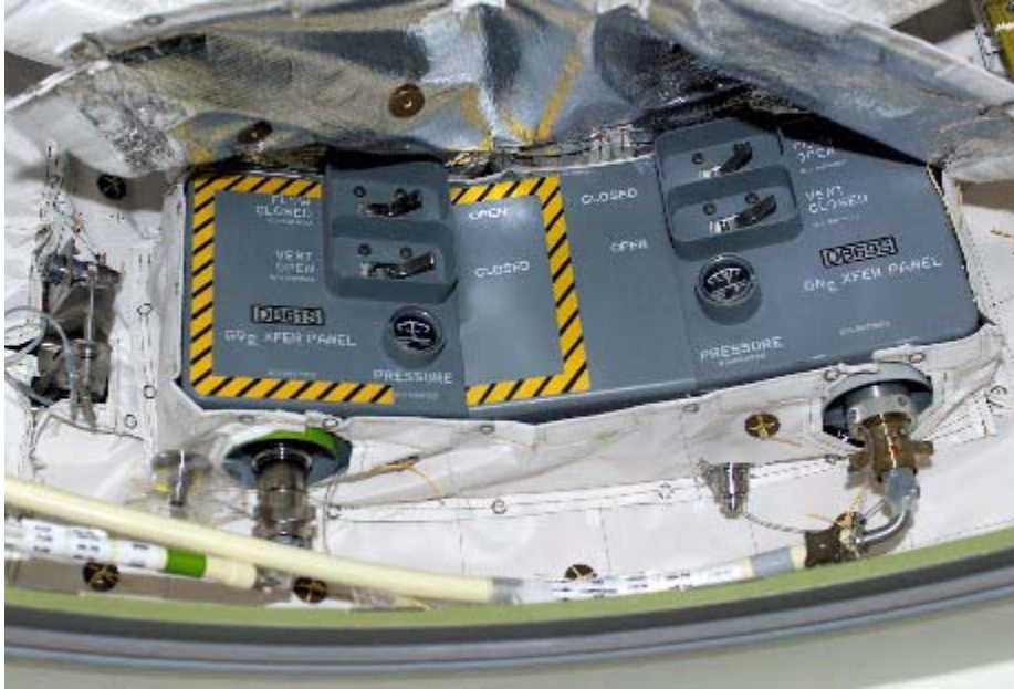
Figure 1.- ODS Vestibule Xfer Panel Hose Routing.
