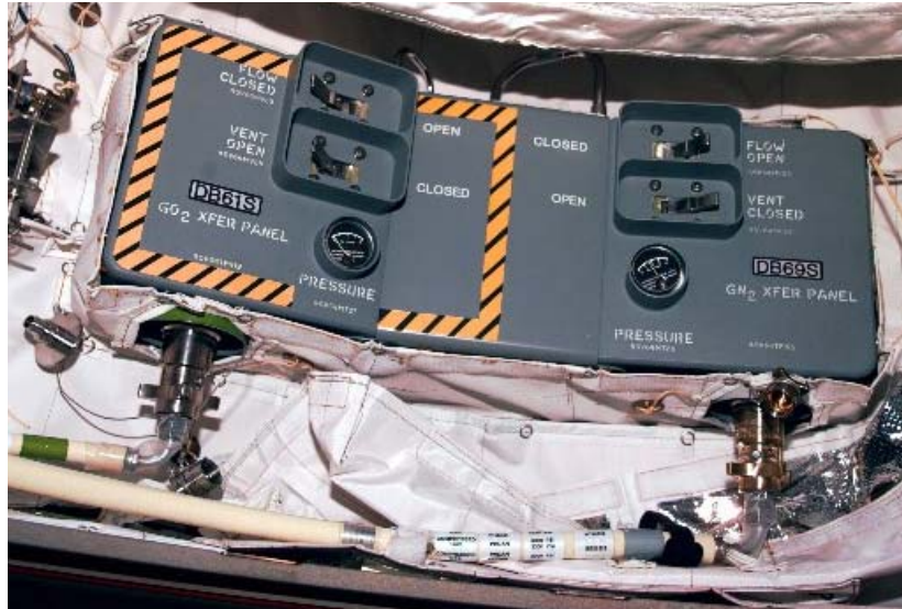
Figure 1.- ODS Vestibule Xfer Panel Hose Routing.
