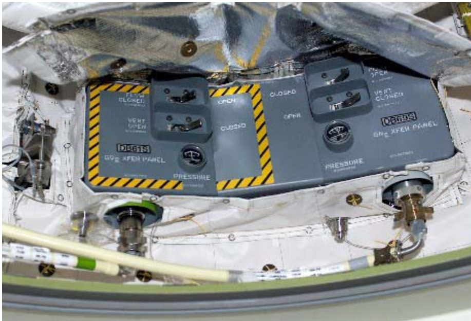
Figure 1.- ODS Vestibule Xfer Panel Hose Routing.
